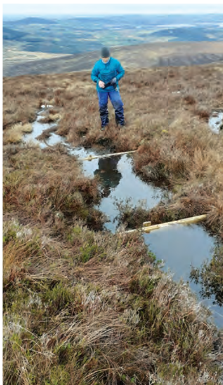
Construction of wooden dams to restore water table levels on Granamore Commonage.
