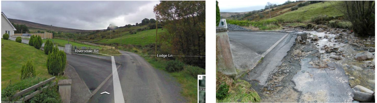
Road washed away by fluvial flooding , before and after
