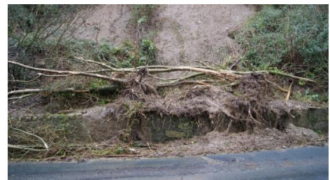
Landslide following heavy rainfall Enniskerry
